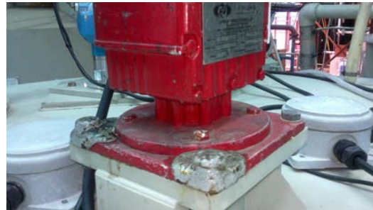
Oxifree coating after exposure to operating environment for 10 months.
