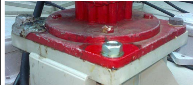
Oxifree coating peeled off from the nut on the right front of the agitator. Compare to the corroded nut at the back, right. Nuts made of stainless steel.
