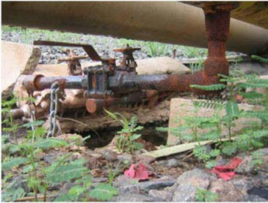
Ball valve with corrosion at its most critical on the elbow connector
